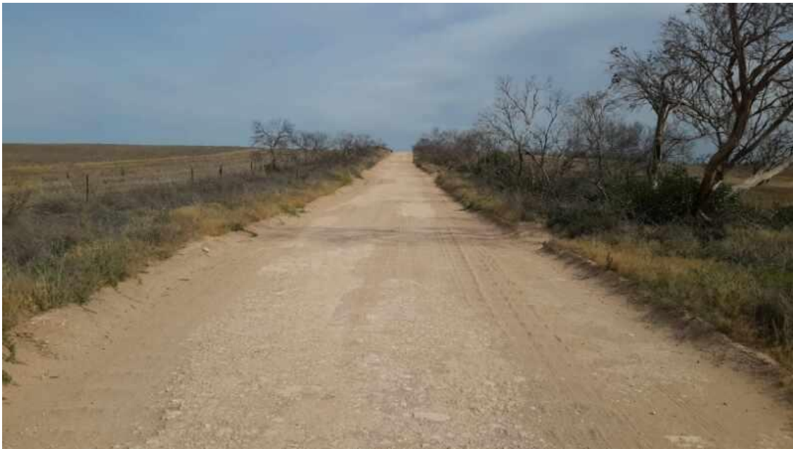
Typical Category 3 Rural Sheeted Road in almost End of Life Condition
