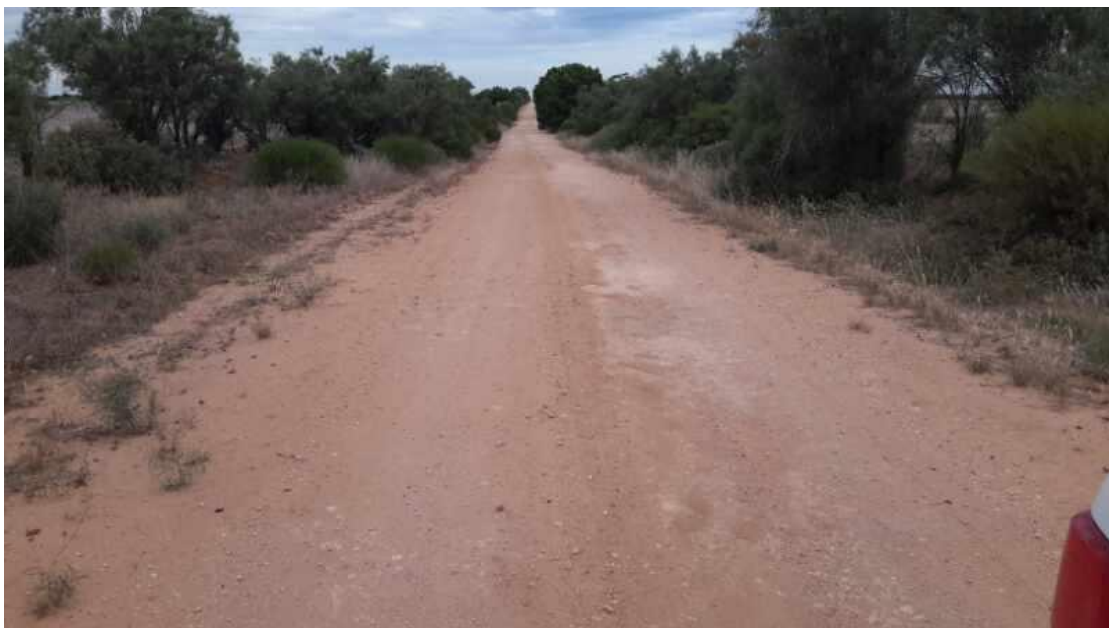
Typical Category 5 Rural Sheeted Road in approaching End of Life Condition
