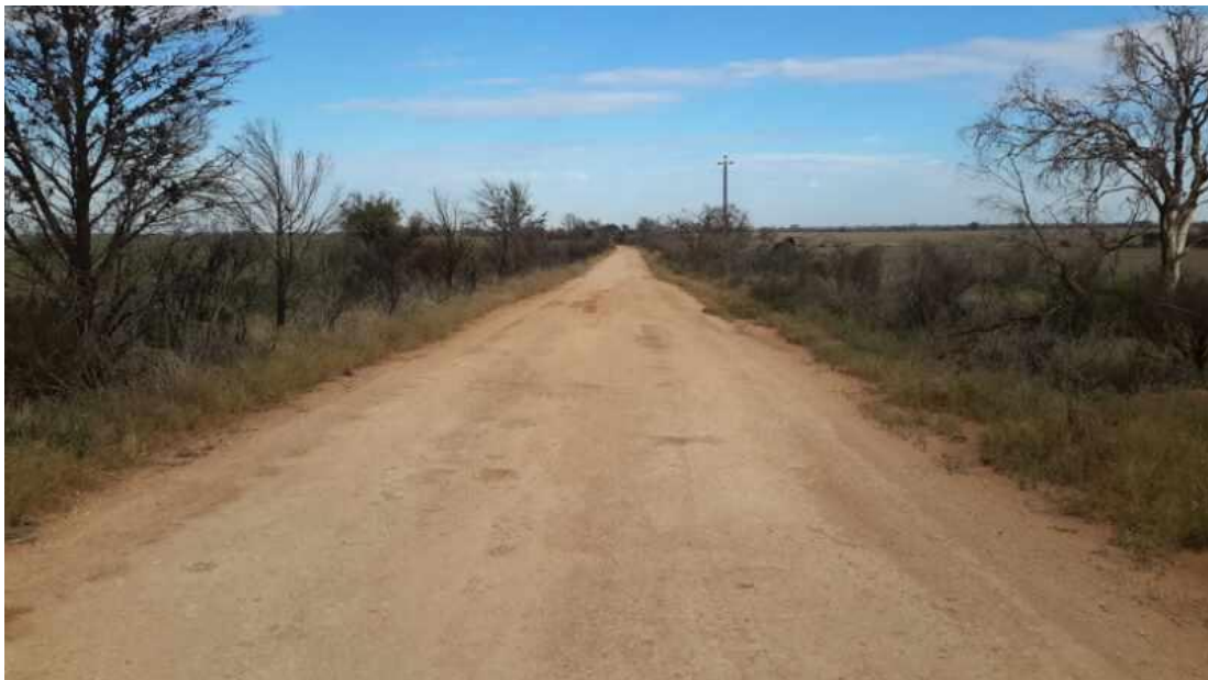
Typical Category 2 Rural Sheeted Road in expired Condition 65
