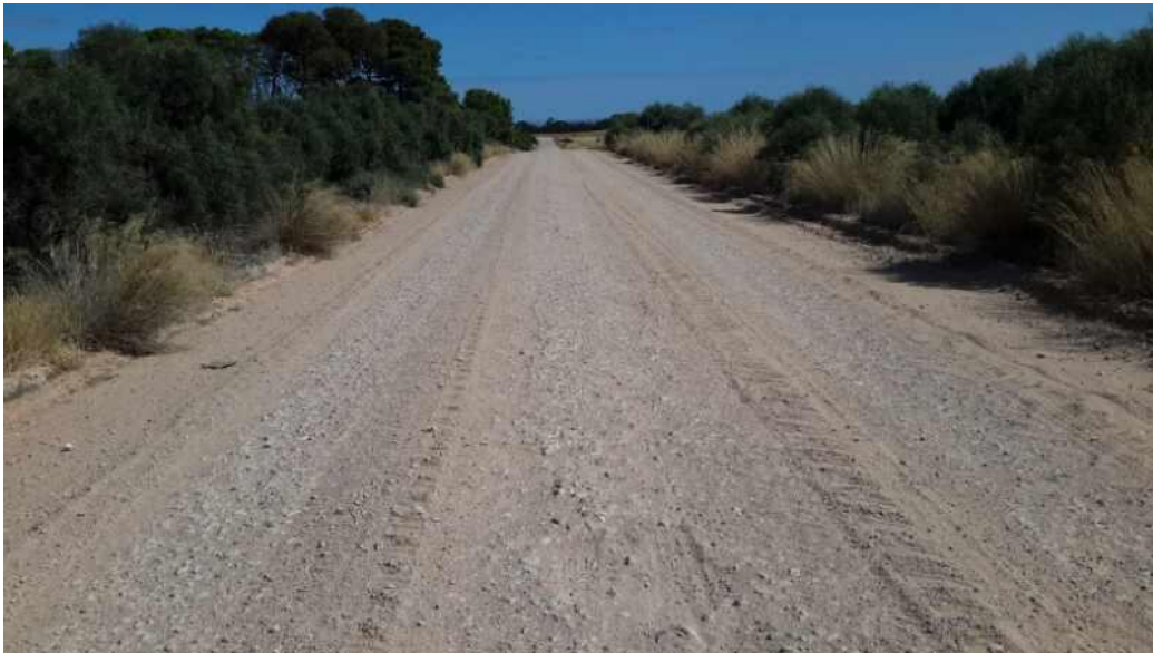
Typical Category 1 Rural Sheeted Road in End of Life Condition 60
