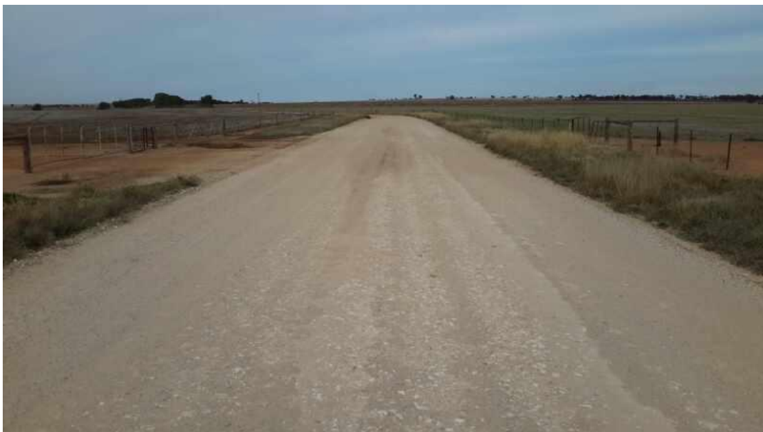
Typical Category 4 Rural Sheeted Road in approaching End of Life Condition 68
