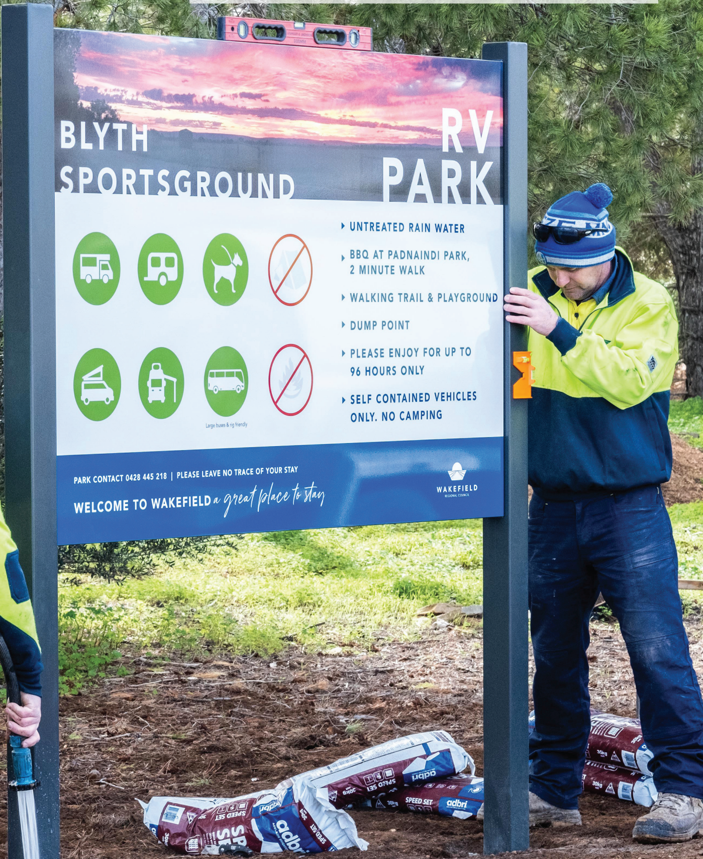
Employees Grant Wilmer and Mitchell Gregory installing a RV Park sign at Blyth.
